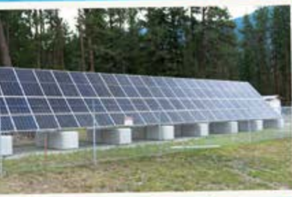
new solar panels
