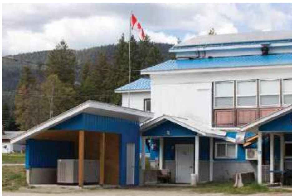
The Legion building in Edgewood, which serves as an emergency readiness centre, now boasts energy upgrades like a generator and a heating, ventilation and air conditioning system.
